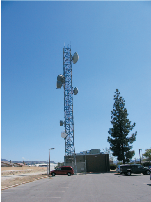
Typical communication tower in an urban setting (Existing county site in Hemet).
